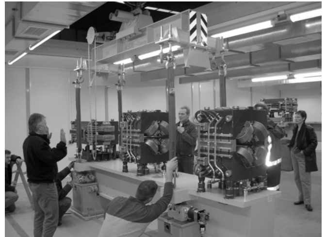
Fig. 2. Girder with traverse, force insertion is in the same position as the stands.
